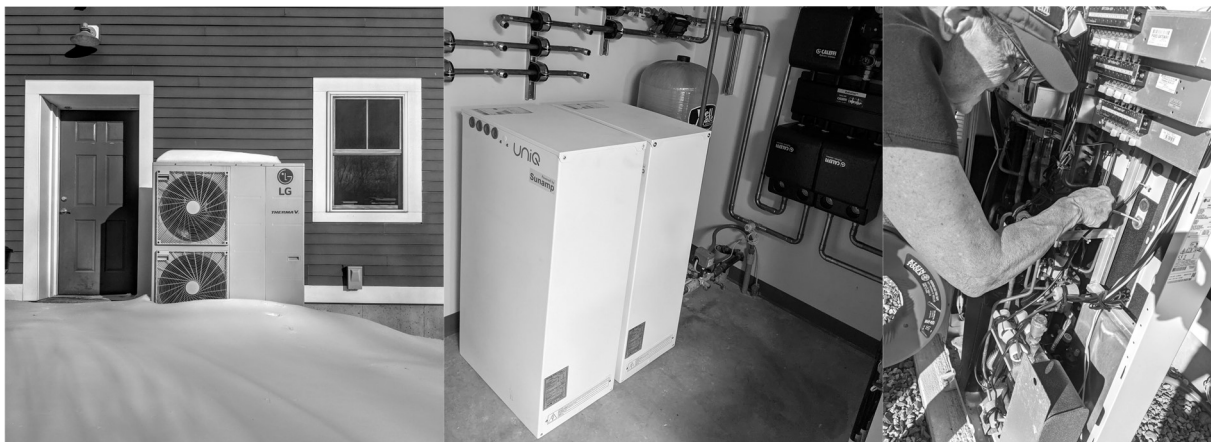
Figure 3: Photos of Type 4 system installed for pilot study in Massachusetts (CZ 5a/6a)
